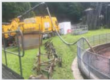
Drainage and empty surface water from PST Tank by a Vacuum Tanker.
