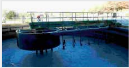
Accumulation of rags on scraper support frame.
