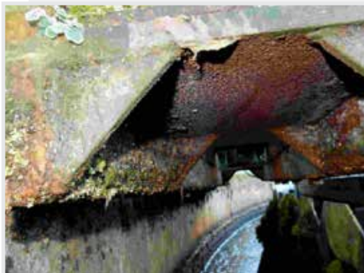
Corrosion on the underside of PST trolley wheel & framework that supports the scraper bridge.
