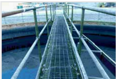
No extensive surface corrosion visible. The scum scraper. Appears to be undamaged.
