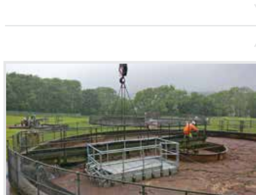
Installation of a floating scaffold making an easy access to the scraper bridge to remove the fixings.
