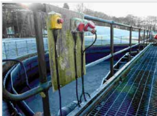
Signs of surface algae growth on metal components.
