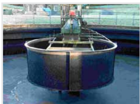
The baffle visibly looks to be in sound condition with no cracks or delamination's.
