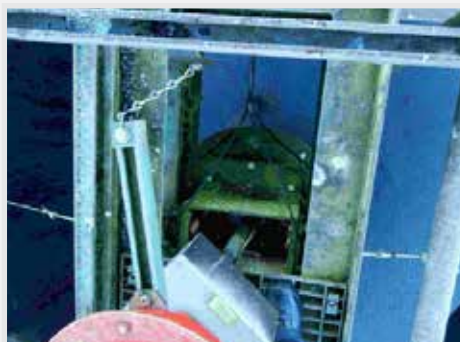
No decking or cover around centre spindle.
