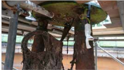
Accumulation of rags on cables loop.
